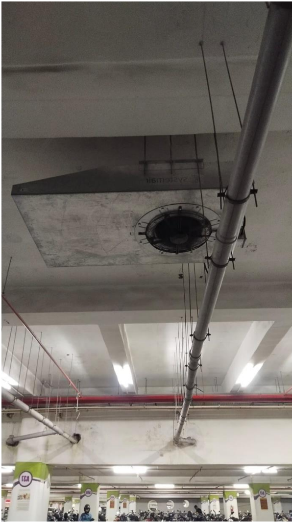
Fig:10 mechanical vent
