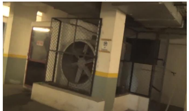
Fig: 17 Mechanical vents
