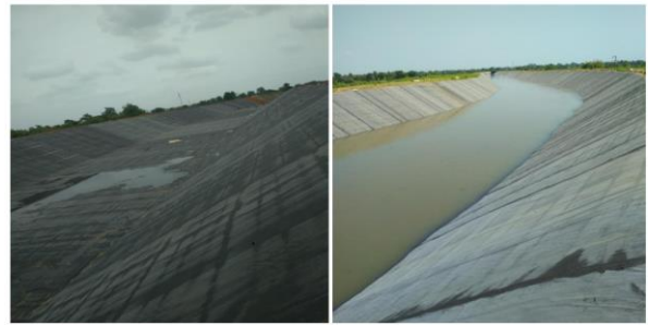
Fig 4: Condition of Canal in July 2019
