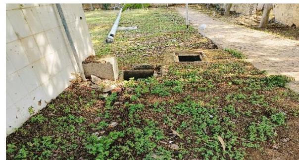
Fig. No. 17: Septic Tanks at the Palkhi Tal
