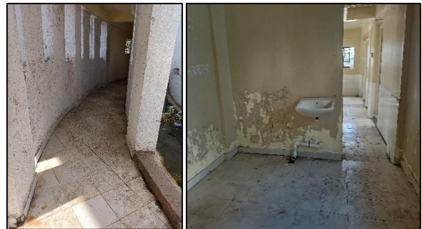
Fig. No. 16: No Proper maintenance of toilets at Palkhi Tal
